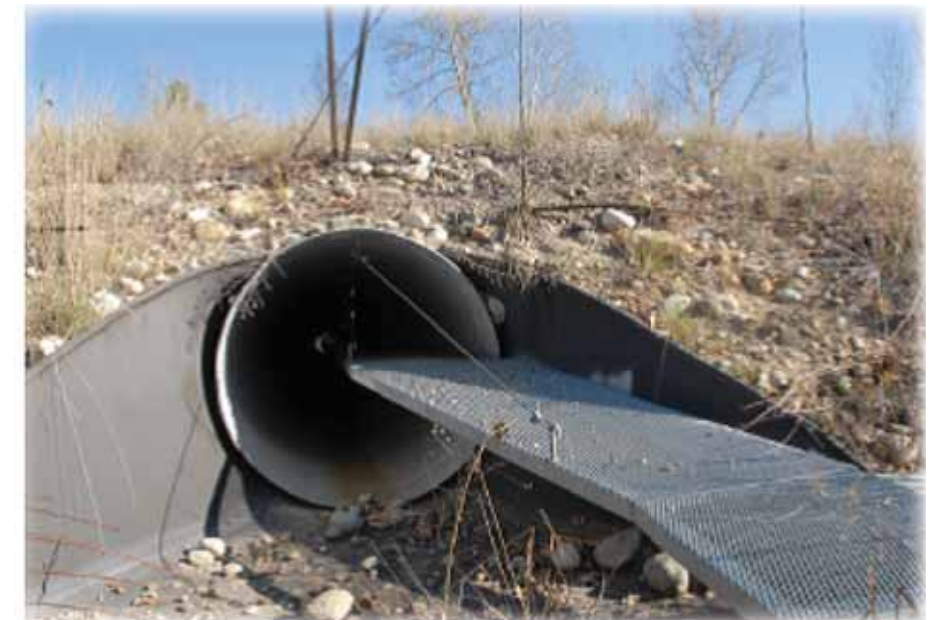
A dry shelf installed in a culvert provides passage for small to medium-sized mammals during periods of high flow. (Image of Critter-Crossing™ Technology)
